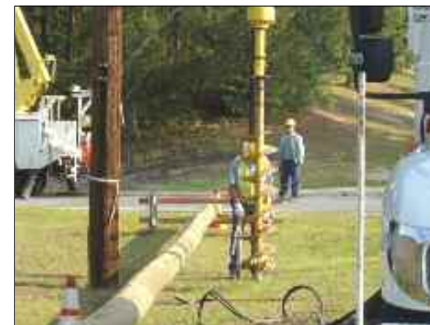
Pictured above and at bottom right, EMEPA crews replace defective poles on the Navy Base.
