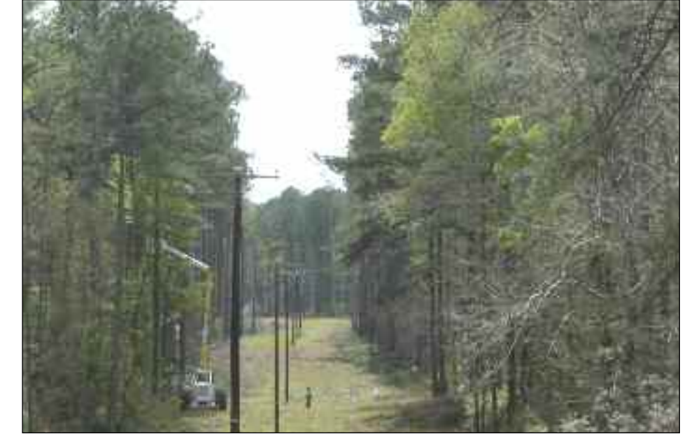
Clearing rights of way has cut down outage time at NAS Meridian.
